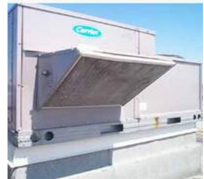
Carrier economizer intake hood
